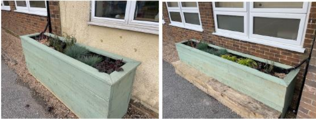
Fig. 9. Images show SuDS rain -planters 3. & 4. on main classrooms.
